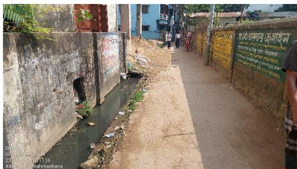
Drain-005, Brahmanbaria Paurashava
